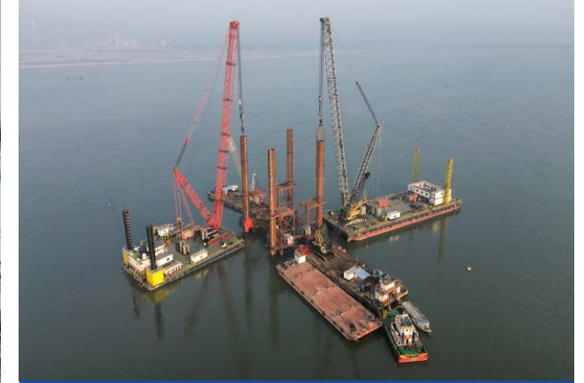
River crossing Transmission Line Project (Bangladesh)
