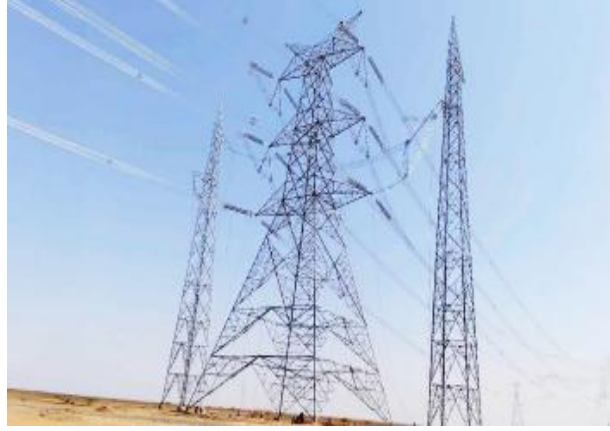
765 kV D/C Transmission lines in Khavda
