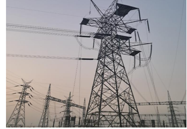
400kV S/C Transmission Line, Rooppur- Bogura (Bangladesh)
