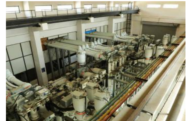
220kV/33kV GIS Substation, Dholera
