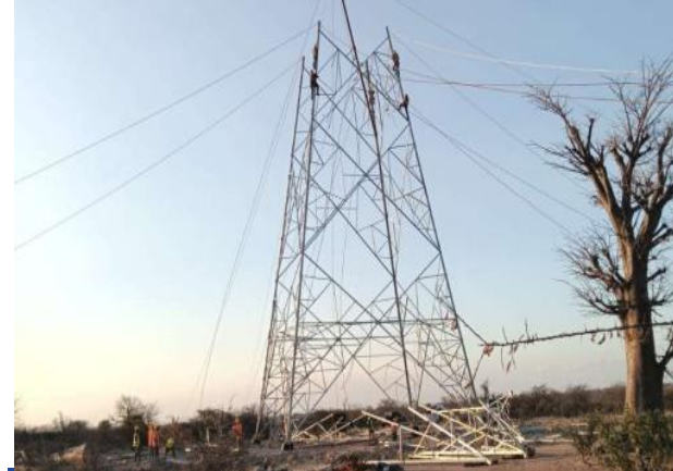
400 kV D/C Transmission Line TaZa Project (Tanzania)
