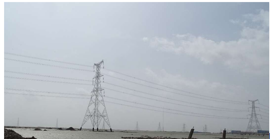
765 kV D/C Transmission lines in Khavda
