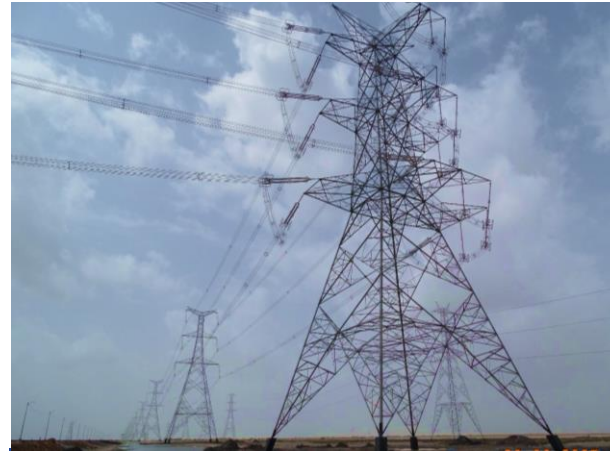
765 kV D/C Transmission lines in Khavda
