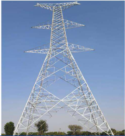
Koppal-II PS – Narendra (New) 765 kV D/C line
