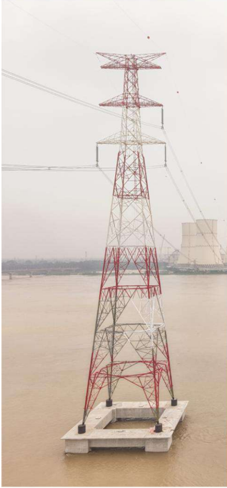
400kV D/C Rooppur-Gopalganj Transmission Line, Bangladesh
