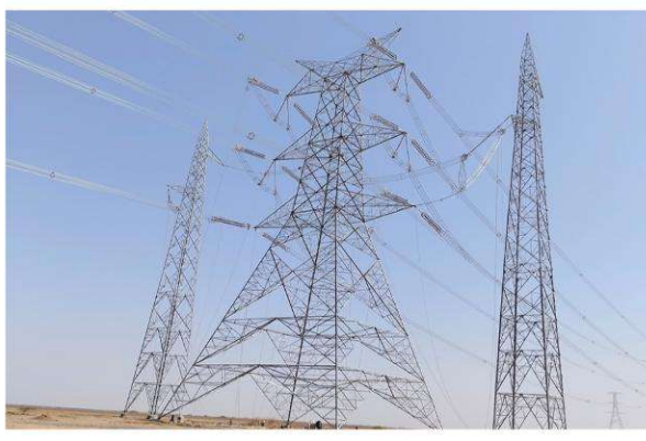
765 kV D/C Transmission lines in Khavda, Gujarat
