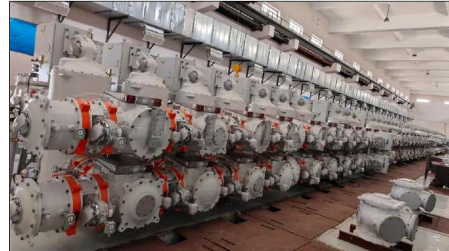
Gas Insulated Substations (GIS)
