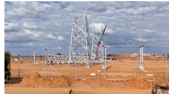
Mmamabula 400 kV substation, Botswana
