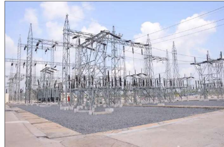
Air Insulated Substations (AIS)
